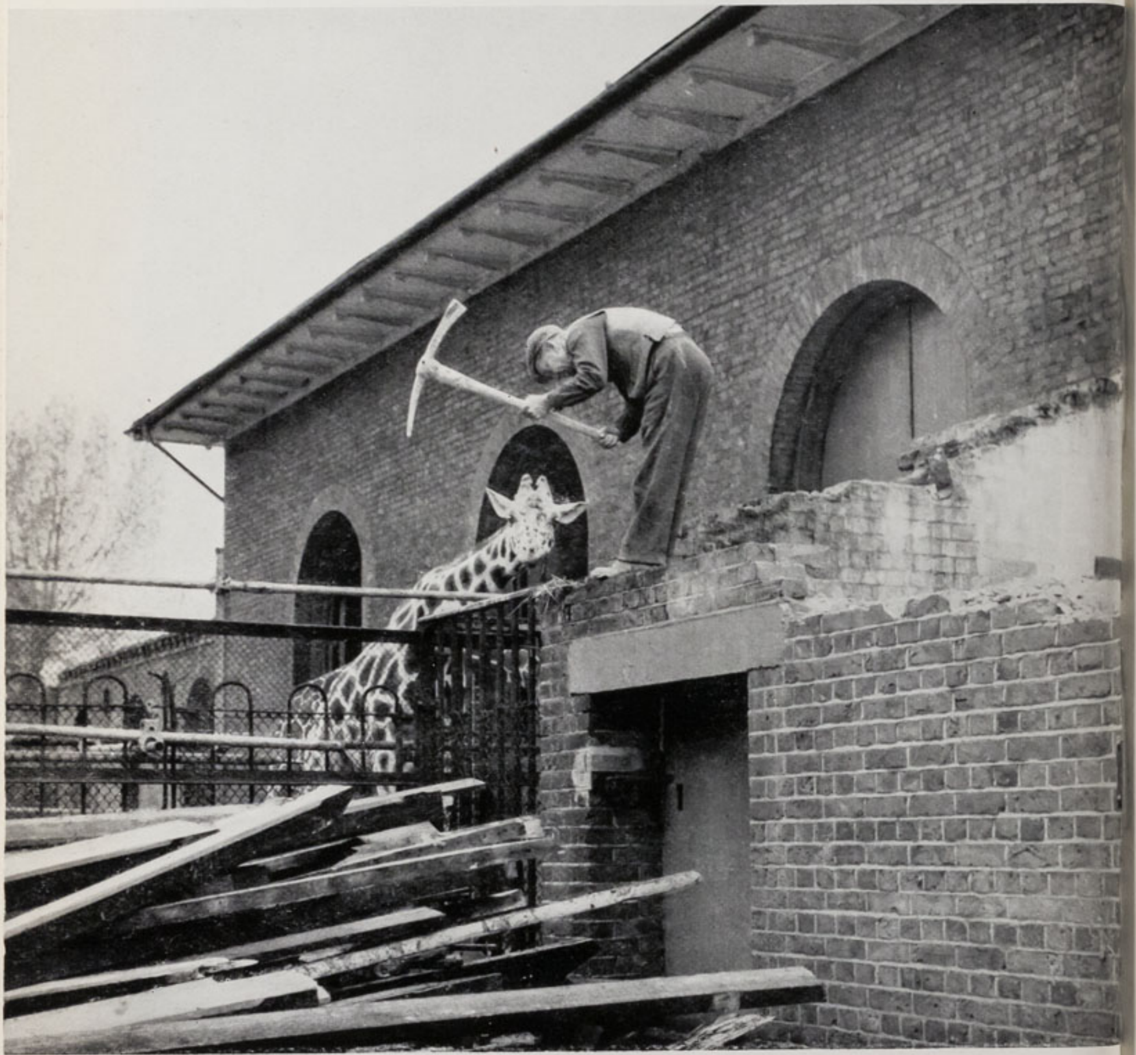
Giraffe watches with interest the demolition of the wing of the Giraffe House.
